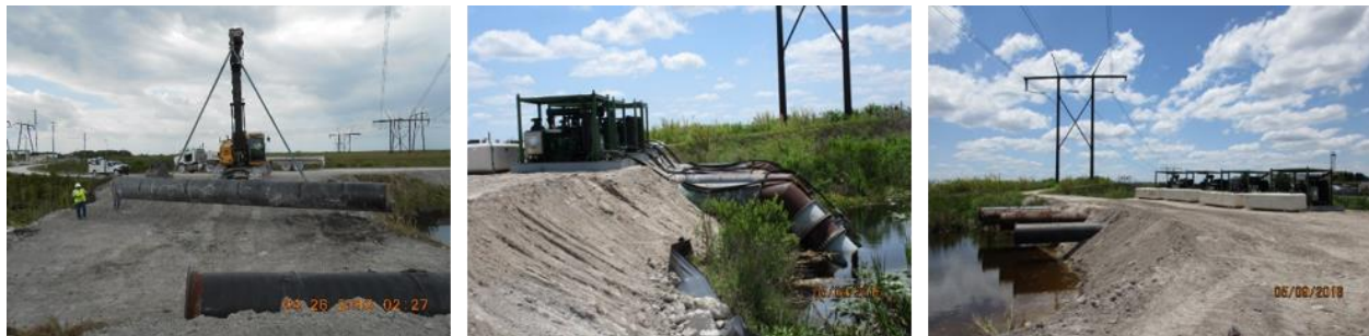
Figure 8. Temporary pumps assembly, intake, and discharge near S-7.
