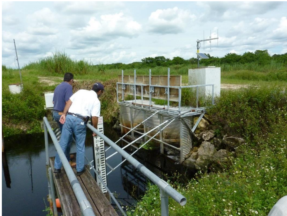
Figure 21: PC-17A Control Structure
