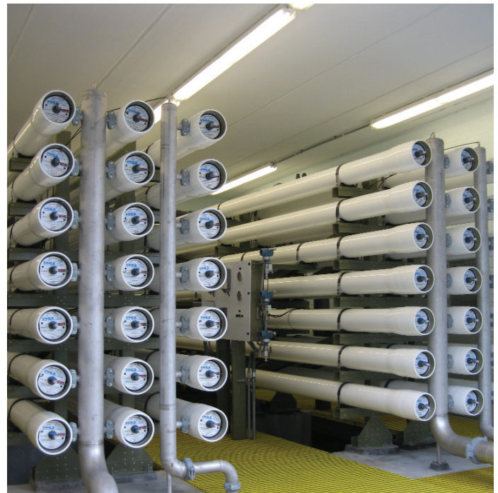
The State of Florida is committed to development of alternative water supply projects, like this reverse osmosis facility.
