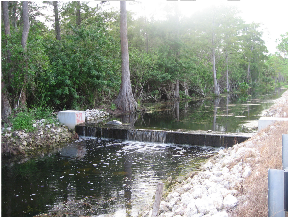
Figure 1-6: San Carlos Estates Moriah Weir with Failed Right Bank Levee
