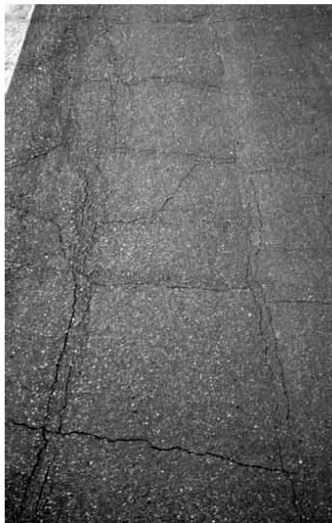
▲ Block cracking with cracks less than 5' apart.
