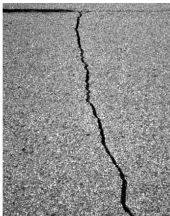
▼ Open cracks need sealing.
