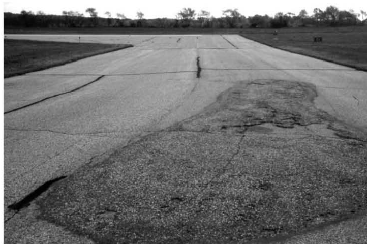
▶ Patch in poor condition.
