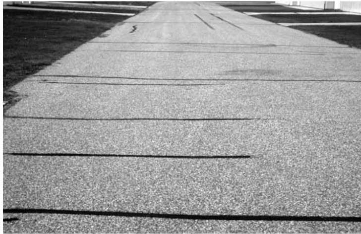
▲ Thermal cracks less than 10' apart. Slight raveling.
