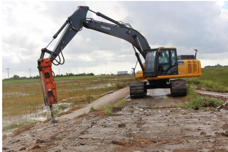
A SFWMD hydraulic ram breaks up the top of the S-327 Weir near Everglades National Park to help send more water to Florida Bay. (Click on the photo for a larger version.)
