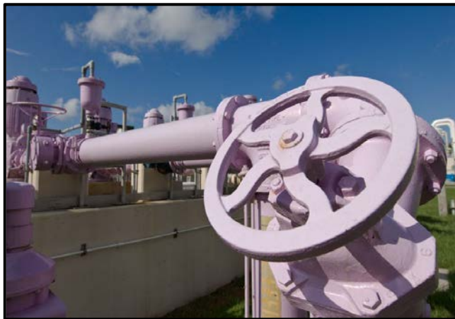
The color purple is used to identify pumps, tanks and pipes carrying reclaimed water.
