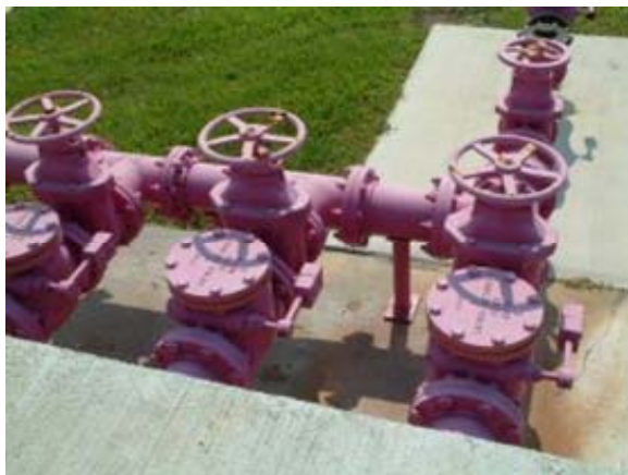
Reclaimed Water Facility
