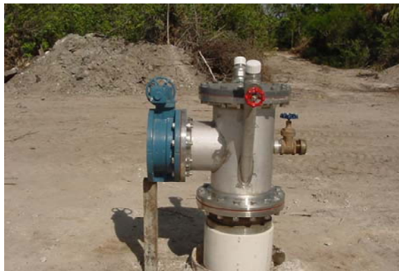
Aquifer Storage and Recovery Well
