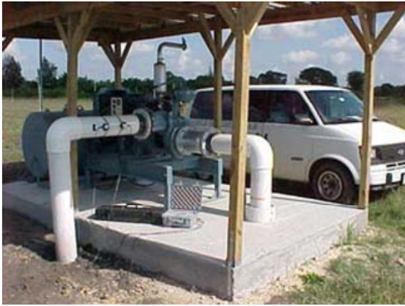
Agricultural Pump Station
