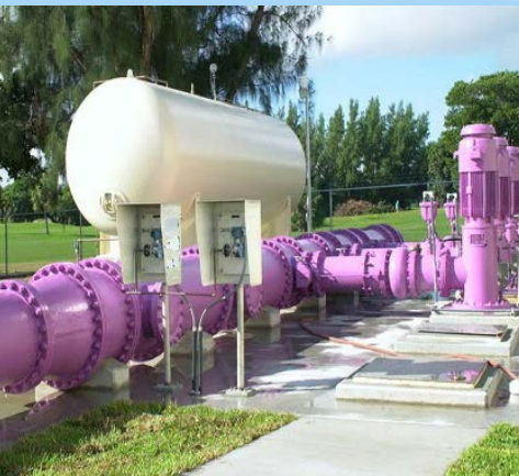
Ensuring Water Supply: Pompano Beach Reclaimed Water Supply Facility
