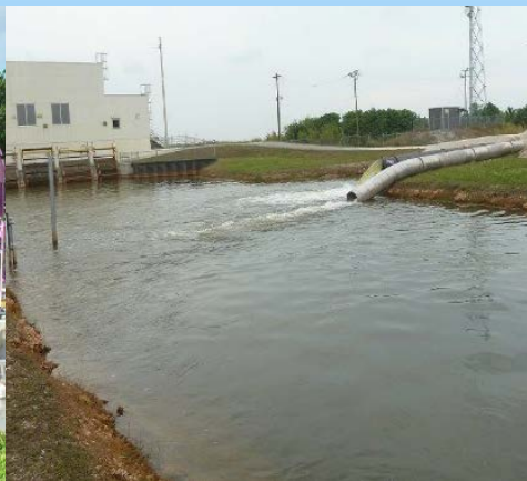
Providing Flood Control: Emergency Operations at S-357 Pump Station
