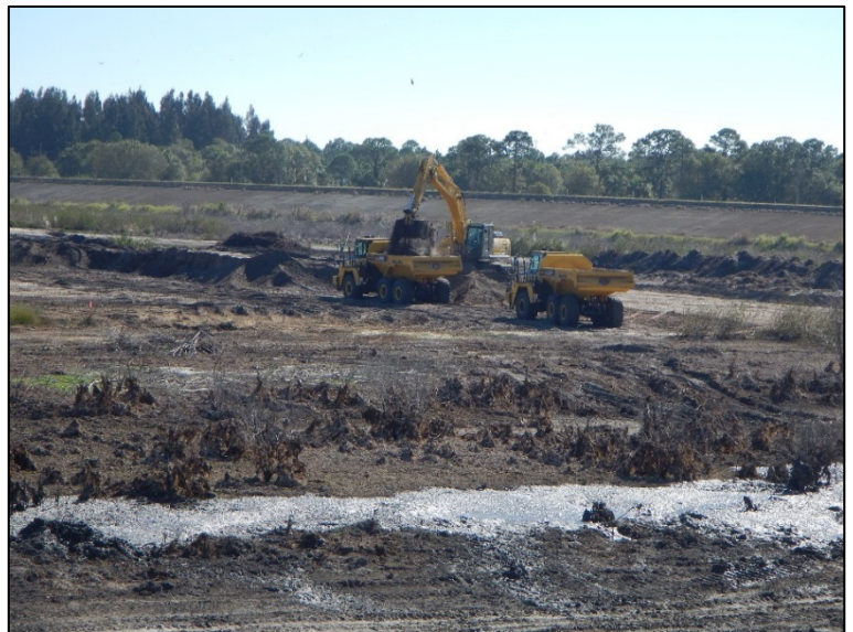
Construction is underway to repair the Ten Mile Creek project in St. Lucie County
