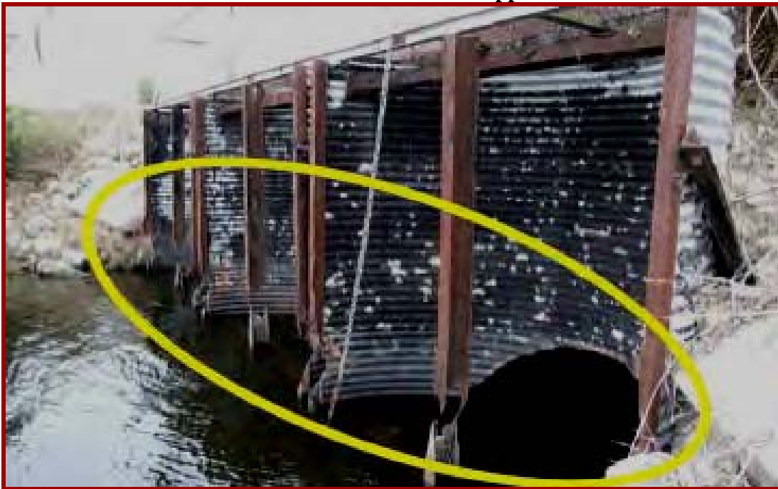
S-39A Culvert Rusted Platform Support
