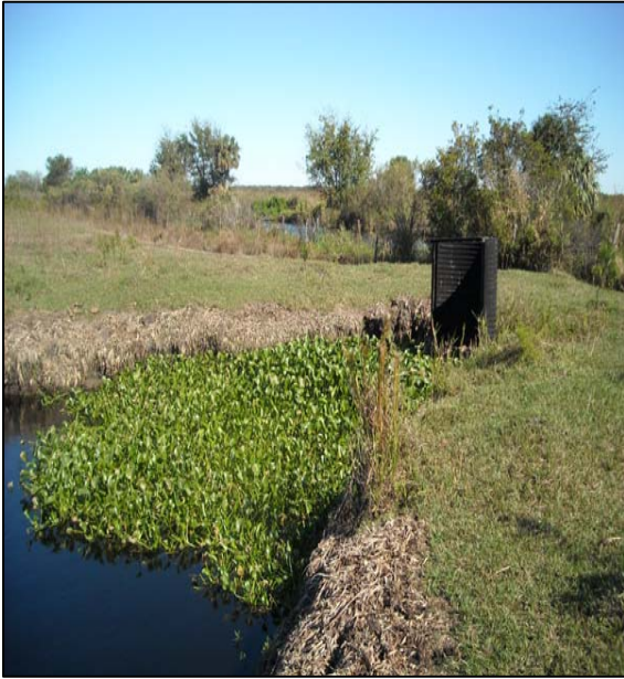
Figure 12. A Culvert Discharging to FEC at the Upstream of Check Dam No.1 Structure (27.27513 N, 81.47126 W)
