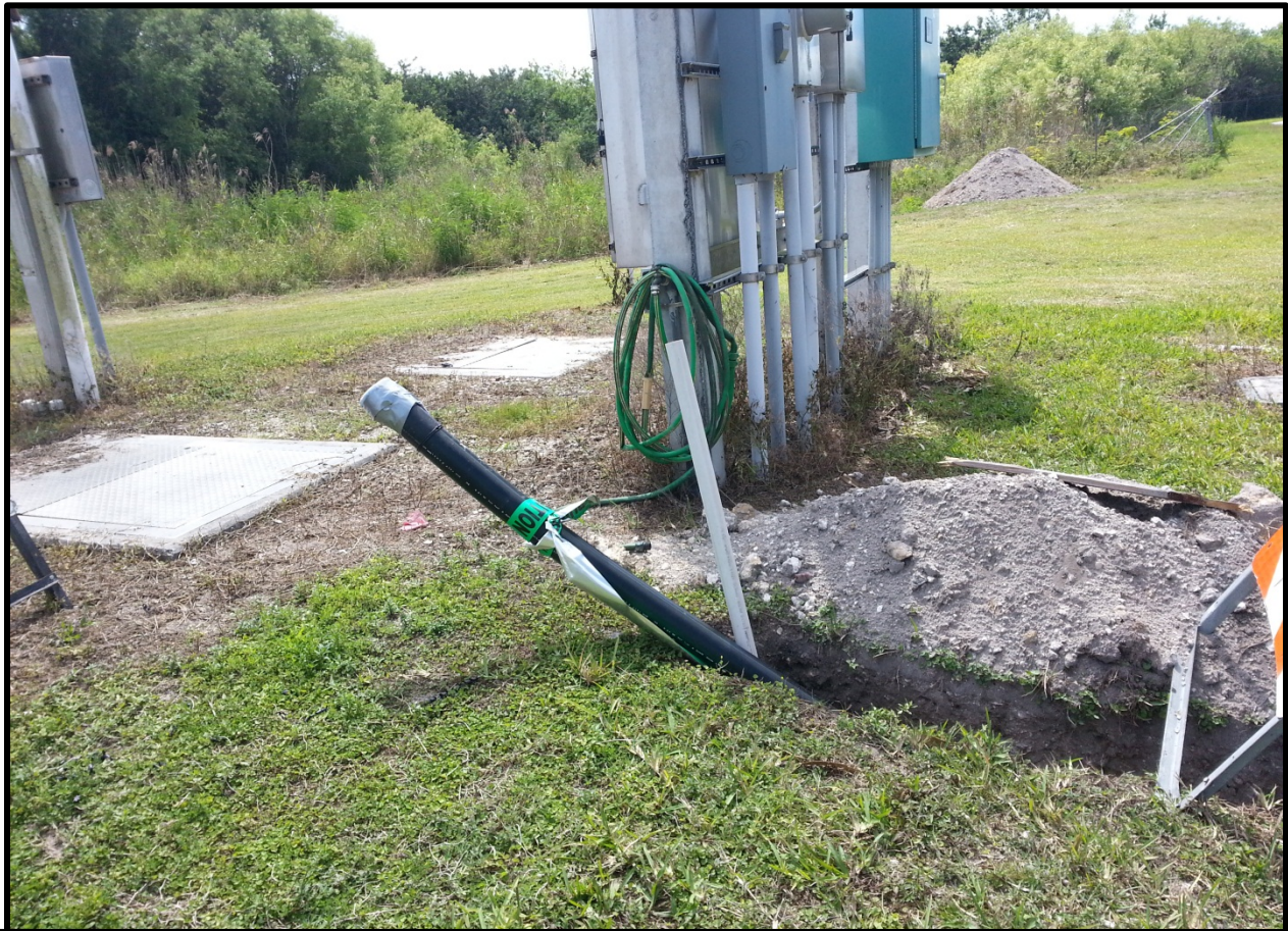
Underground concentrate piping between water plant and wastewater treatment plant. Observed March 19, 2014.
