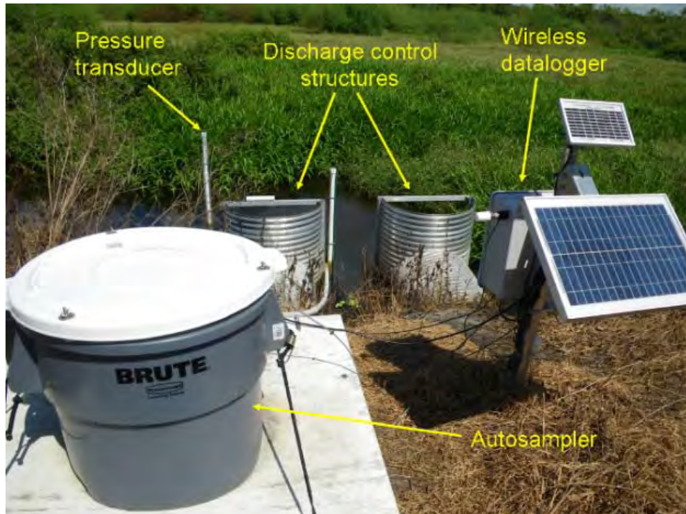
Figure 12. Surface water quantity and quality monitoring system installed at the discharge site.
