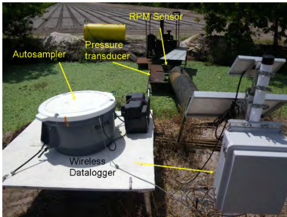
Figure 9. Surface water quantity and quality monitoring system installed at pump 1
