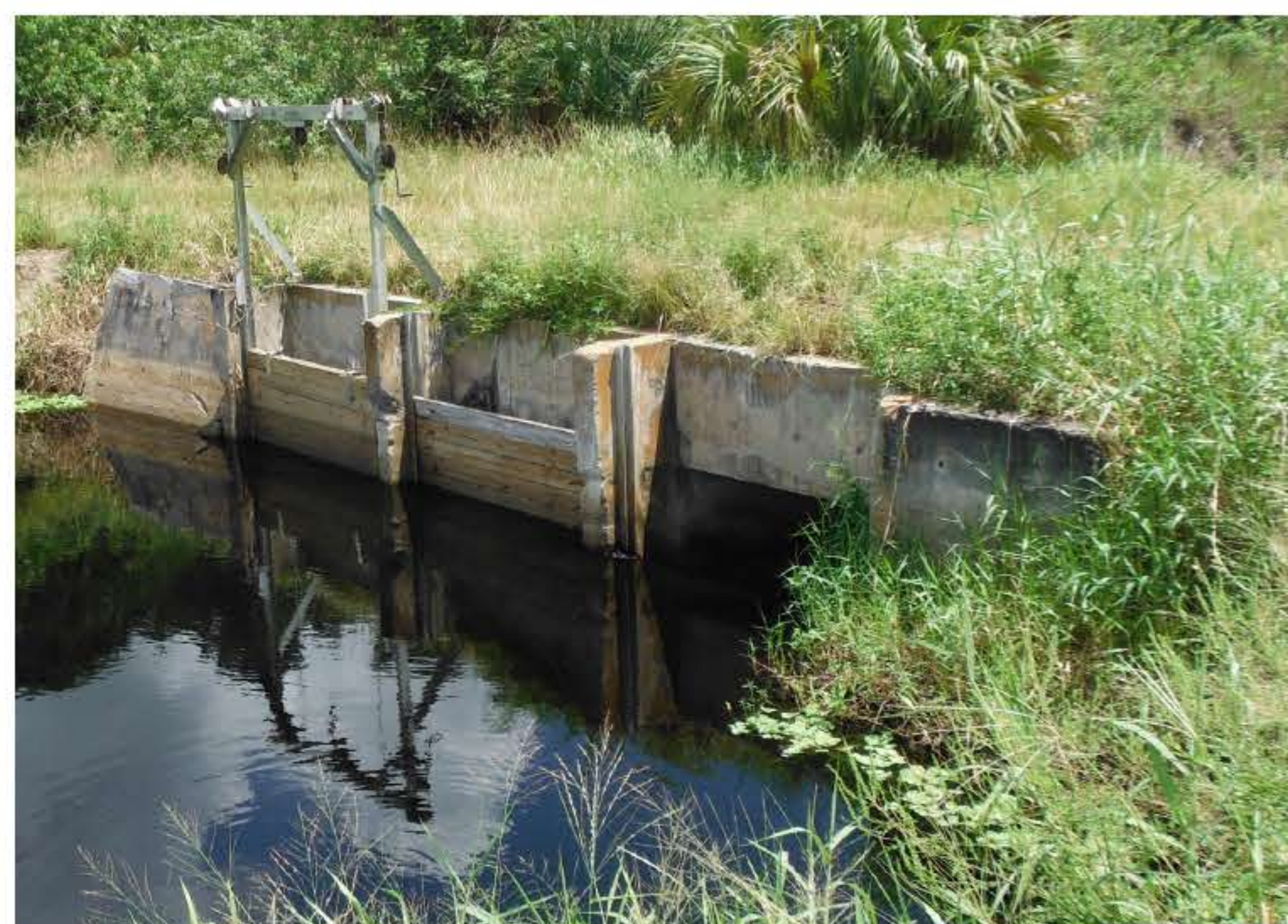
Use of Risers to Reduce Discharge
