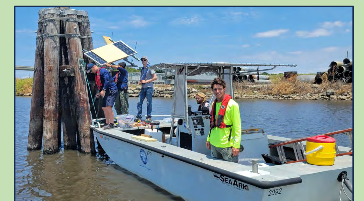
S-308C channel marker on Lake Okeechobee. Installing solar panels to power the deployed continuous monitoring equipment.
