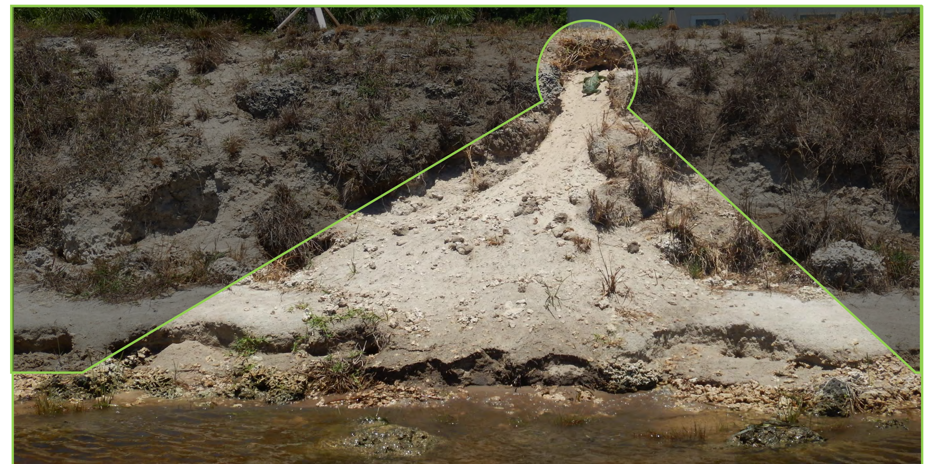
Figure 4 . Iguana burrows in the sides of levees increase erosion.
