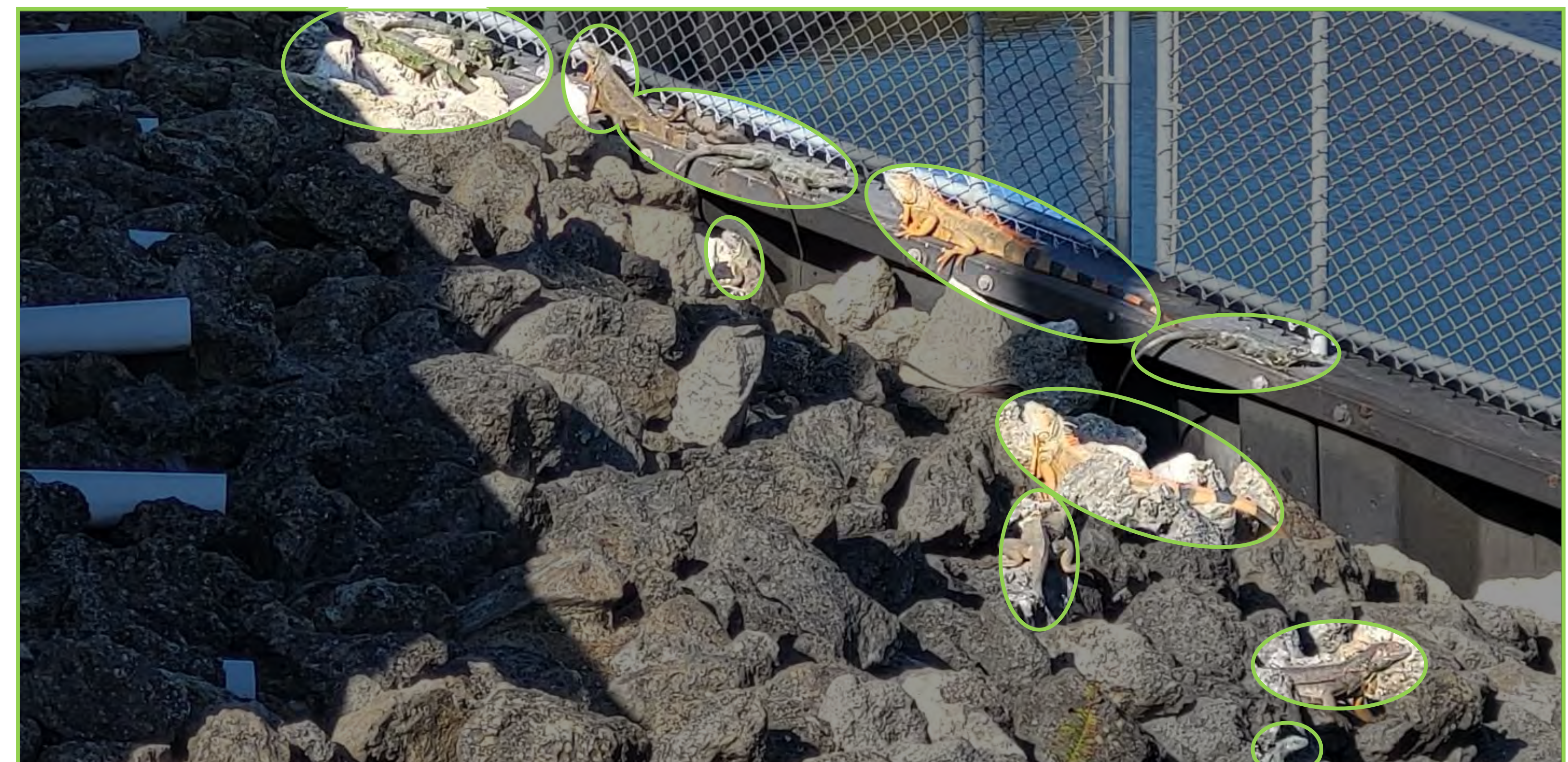
Figure 5. Riprap used to reinforce levees creates habitat for iguanas to utilize and burrow beneath.
