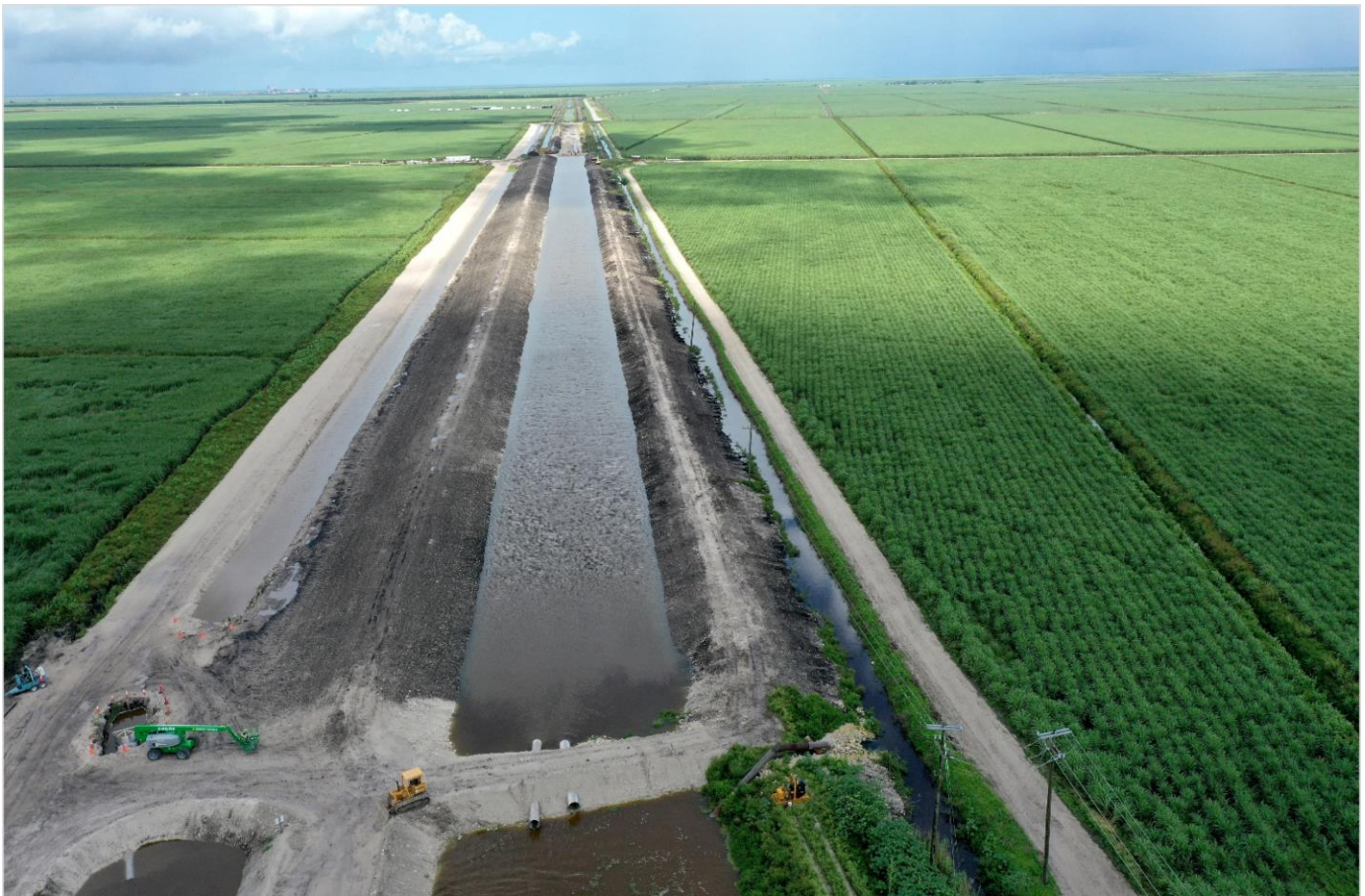
Westward view of a completed portion of Segment 4 in the Bolles East Canal as part of the G-341 Conveyance Related Improvements. Berms awaiting hydroseeding.
