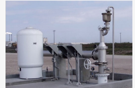
Clewiston Injection Well
