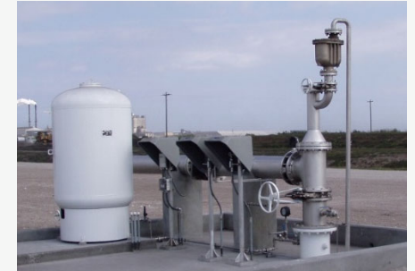
Clewiston Injection Well
