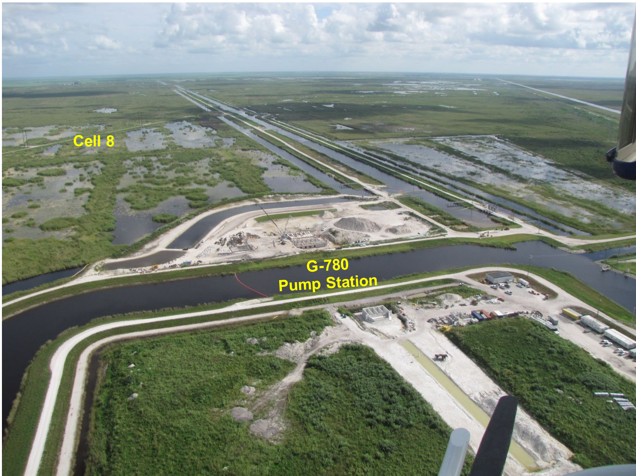
Aerial view of STA-1W Cell 8 and the G-780 Pump Station under construction. Image is facing north
