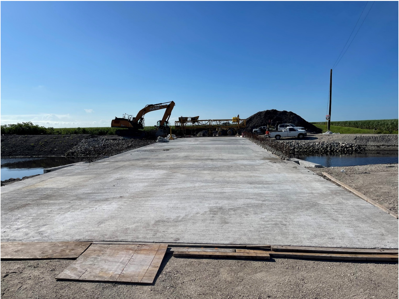
Construction of the Boca Chica Bridge. Substantial completion is expected by mid November.
