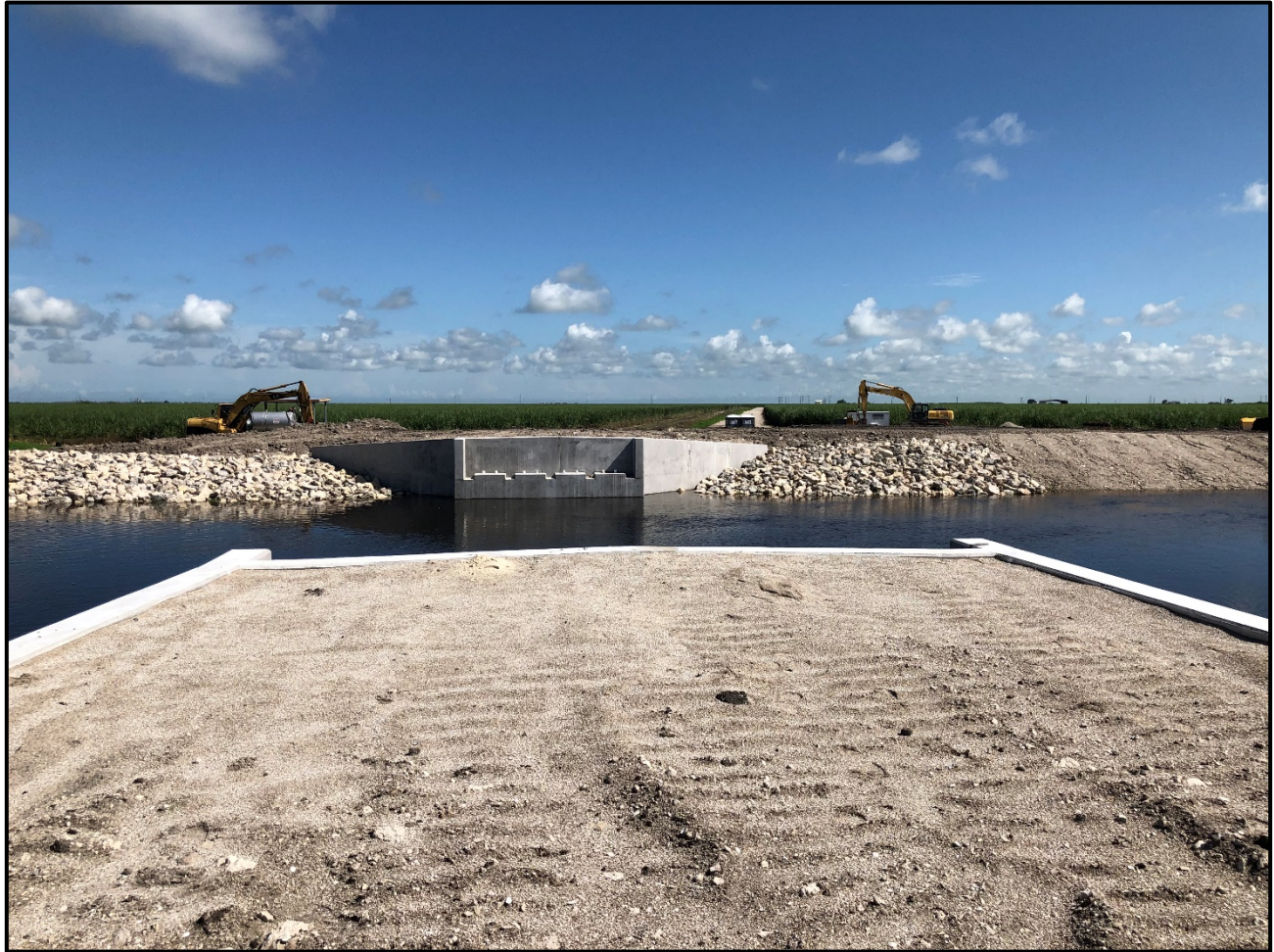
G-341 Related Conveyance Improvements: Bridge supports of the JET Farms Bridge awaiting the delivery of the steel superstructure.
