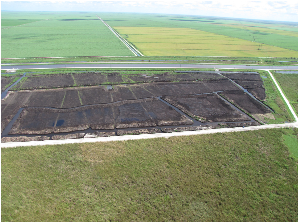
Aerial view of the STA-2 Refurbishment Project. Image shows the regrading activities in the northeast portion of Cell 2.
