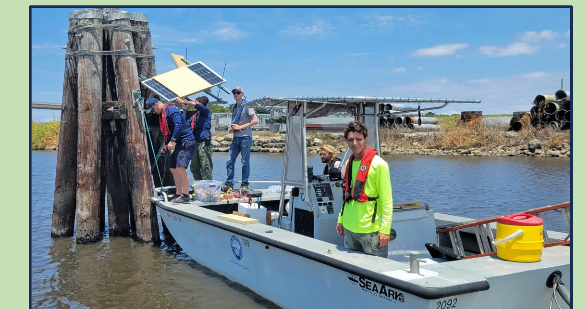
S-308C channel marker on Lake Okeechobee. Installing solar panels to power the deployed continuous monitoring equipment.
