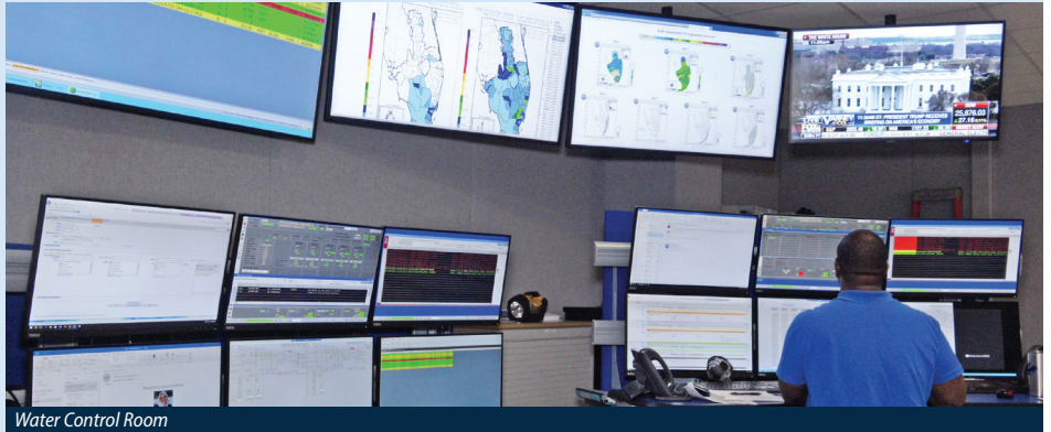
Water Control Room
