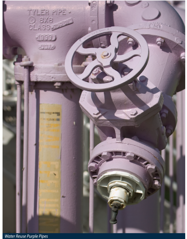
Water Reuse Purple Pipes
