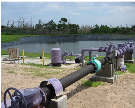
Reclaimed Storage Pond and Pump Station
