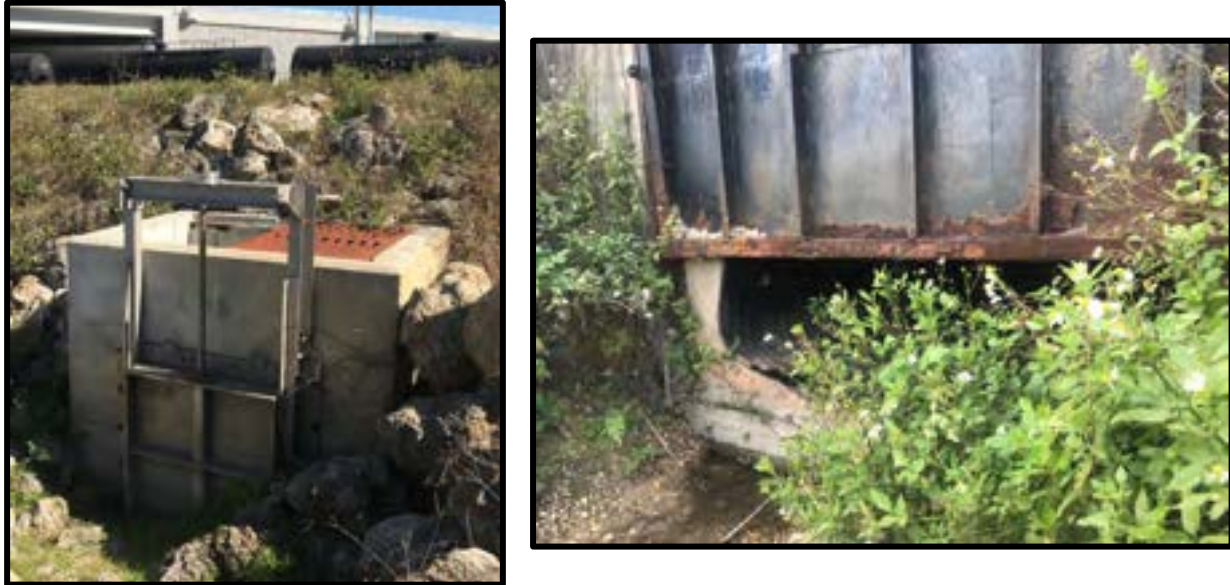
Figure 5 – Existing Canal Interconnect Structures at Carrell Canal (left) and IDD Canal L (right).
