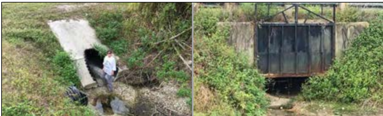
Figure 9. Photos of the Culvert and Gate Structure Connecting L Canal and Ten-Mile Canal
