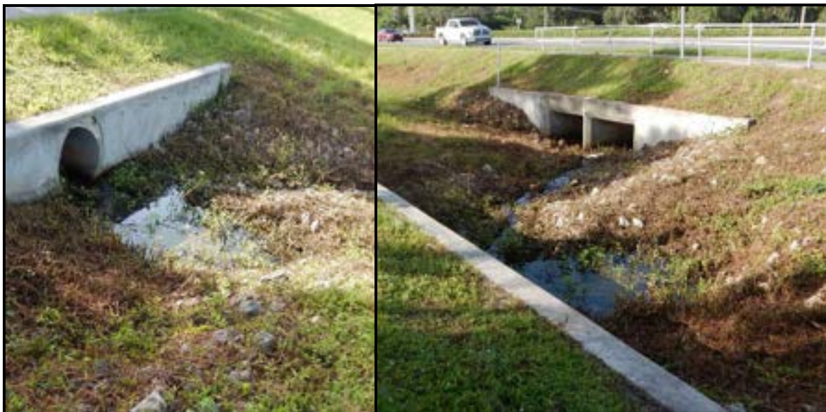
Figure 10 - Existing culverts in Canal J under the east frontage road (left) and US 41 (right).
