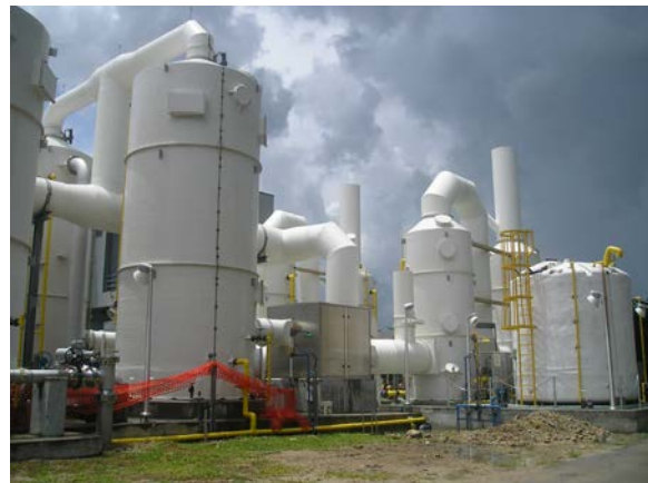
Water Treatment Plant in Collier County
