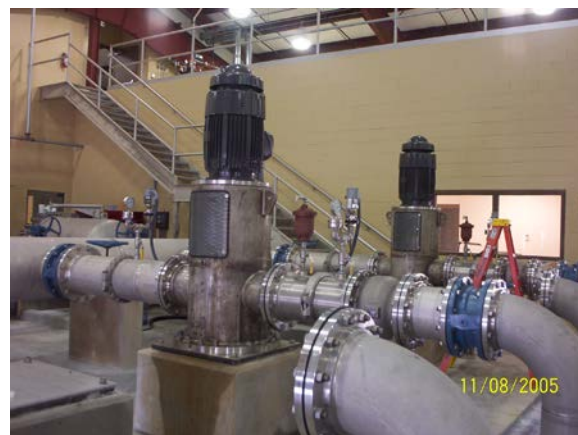
Water Treatment Facility – Pumps to Membrane Trains
