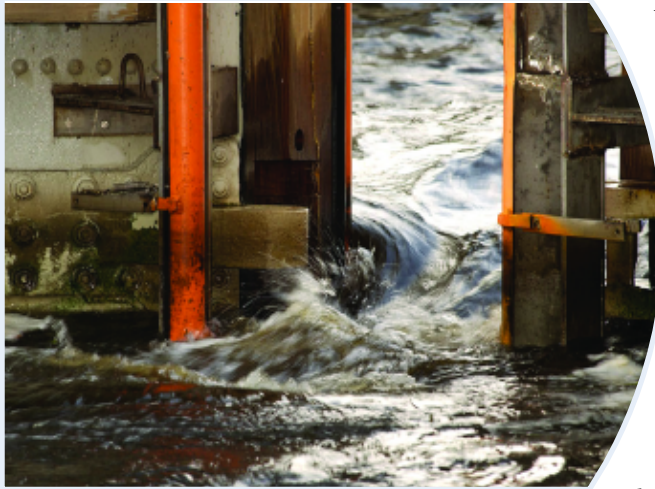
The S-193 structure lock opening, Lake Okeechobee.
