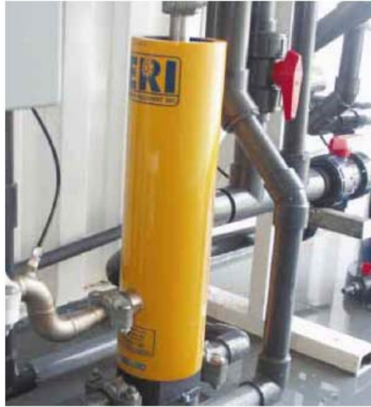
Figure 4.23 – Pressure Exchanger Installation
