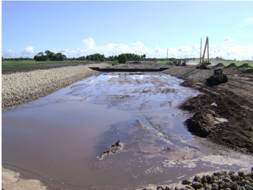
Figure 1. View of the dewatered Nubbin Slough Stormwater Treatment Area S-385 Pump Station Intake Canal for the construction of the upstream weir. May 4, 2012.
