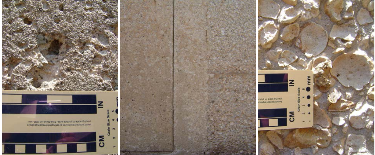
Figure 16. Comparison between the deteriorated concrete surface on the 1970 concrete (left) and the 1935 concrete (right). The 1970 concrete exhibit pits from dissolved limestone fragments while the 1935 concrete exhibits partially dissolved shell fragments in a dissolved cement-fine aggregate matrix. July 31, 2012.
