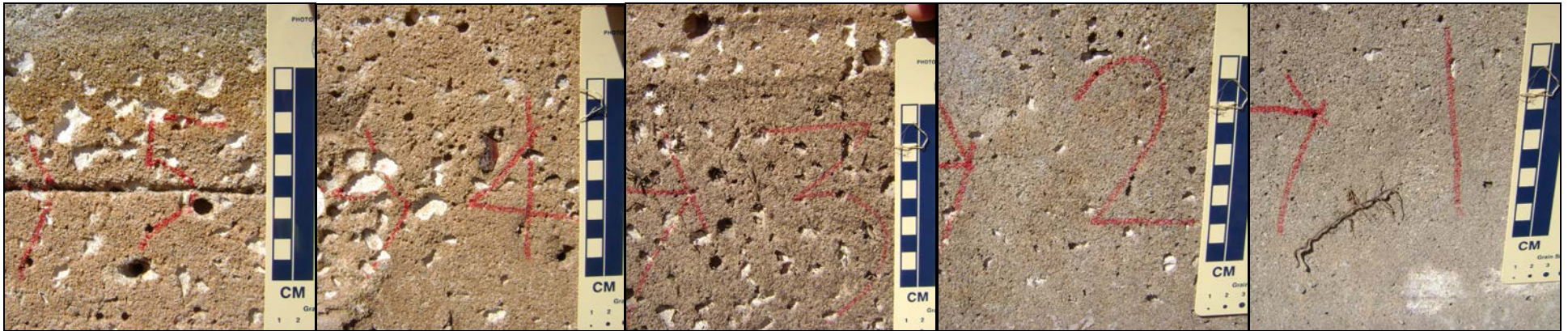
Figure 3. Variation in concrete pitting with water depth at the Nubbin Slough STA S-385 Pump Station. Measurements are at 1-foot intervals from the surface of the concrete slab (+12.0 ft. NGVD29). Concrete pitting diminishes at depth. May 24, 2012.
