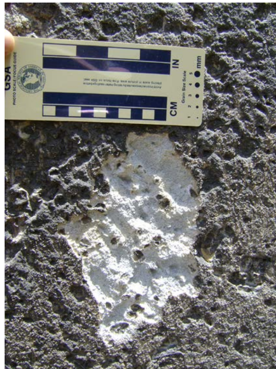
Figure 17. View of the deteriorated S-193 Navigational Lock Structure concrete after scraping the concrete surface with masonry hammer. Take note of the holes which are remnants of the dissolved coarse limestone aggregates from the 1970 concrete. July 31, 2012.
