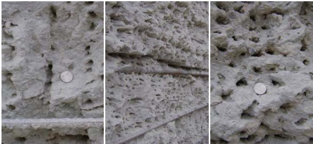
Figure 9. View of the hydroblasted concrete surfaces at the Navigational Lock S-61 Boat Lock indicating deep voids/pits that are aligned resulting from high pressure mechanically-operated hydroblasting equipment.
