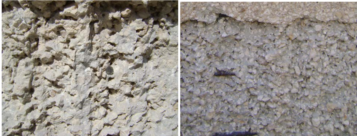
Figure 10. Photographs of the hydroblasted concrete surfaces at the Navigation Lock S-65A showing significant amount of the fine grained concrete matrix being removed thus resulting to deep narrow voids.
