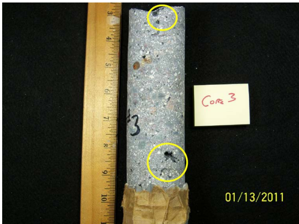
Figure 13. Photograph of a shotcrete core from S-65A Navigational Lock showing 1/16" to 5/8" voids. 41
