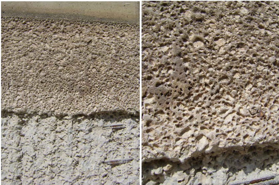
Figure 7. View of the partially hydroblasted concrete surface of the S65D Navigation Lock. The upper portion of the photograph shows the pitted concrete surface. The holes are remnants of dissolved coarse limestone aggregates. August 4, 2010.
