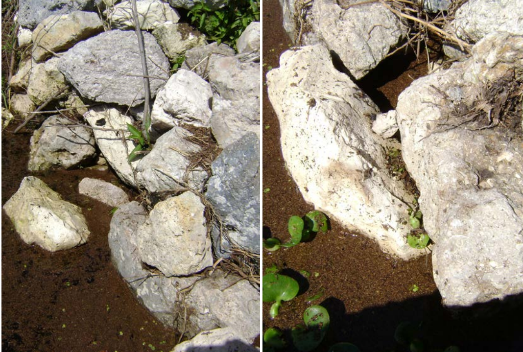
Figure 6. Photographs of limestone rubble riprap located downstream of the Nubbin Slough STA S-385 Pump Station Weir. Take note of the limestone rubble near the water surface showing smooth surfaces which may be attributed to acidic water. May 24, 2012.
