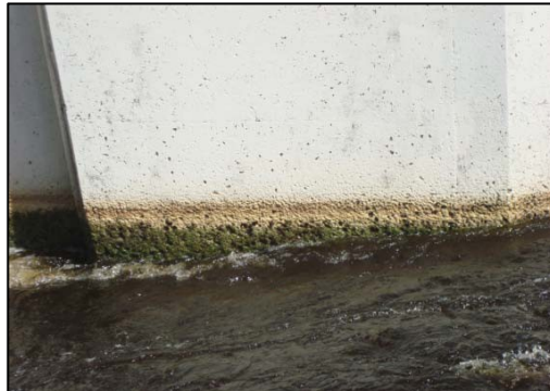
Figure 9. Sulfate Attack on Concrete
