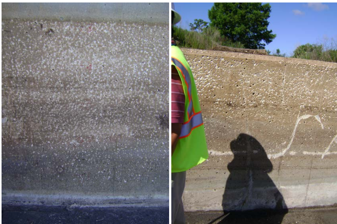
Figure 2. Photographs showing the variation on the extent of deteriorated concrete surface at the Pump Station S-385 intake bay (left) and weir (right). May 24, 2012.
