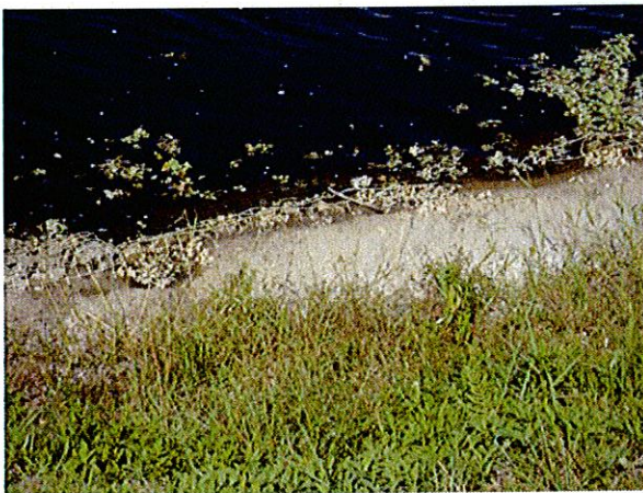
Downstream – North Bank – Failed Gabion
