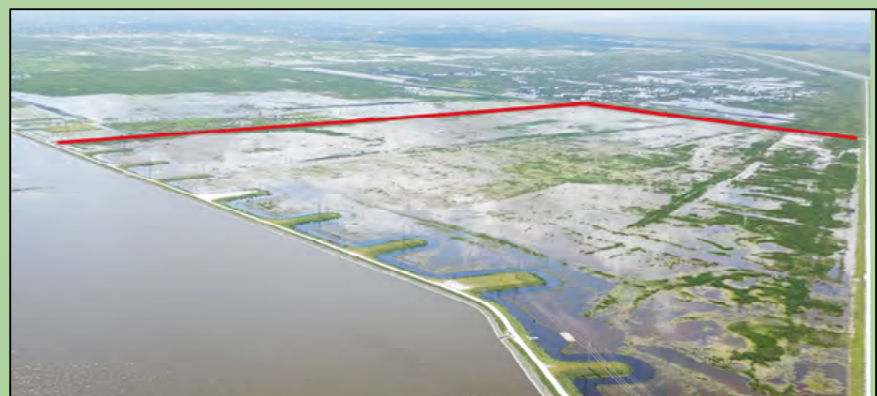
STA-1E Improvements Southwest view of Cell 7. Cells 5 and 7 were regraded to repair differences in elevation
