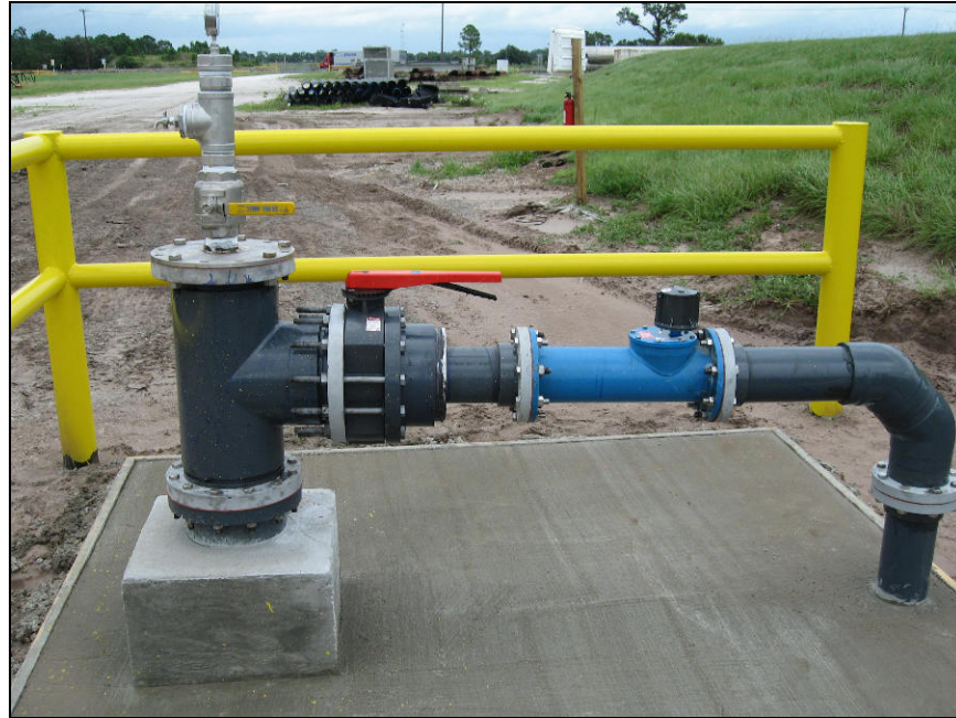
Figure 6. Wellhead and well pad.
