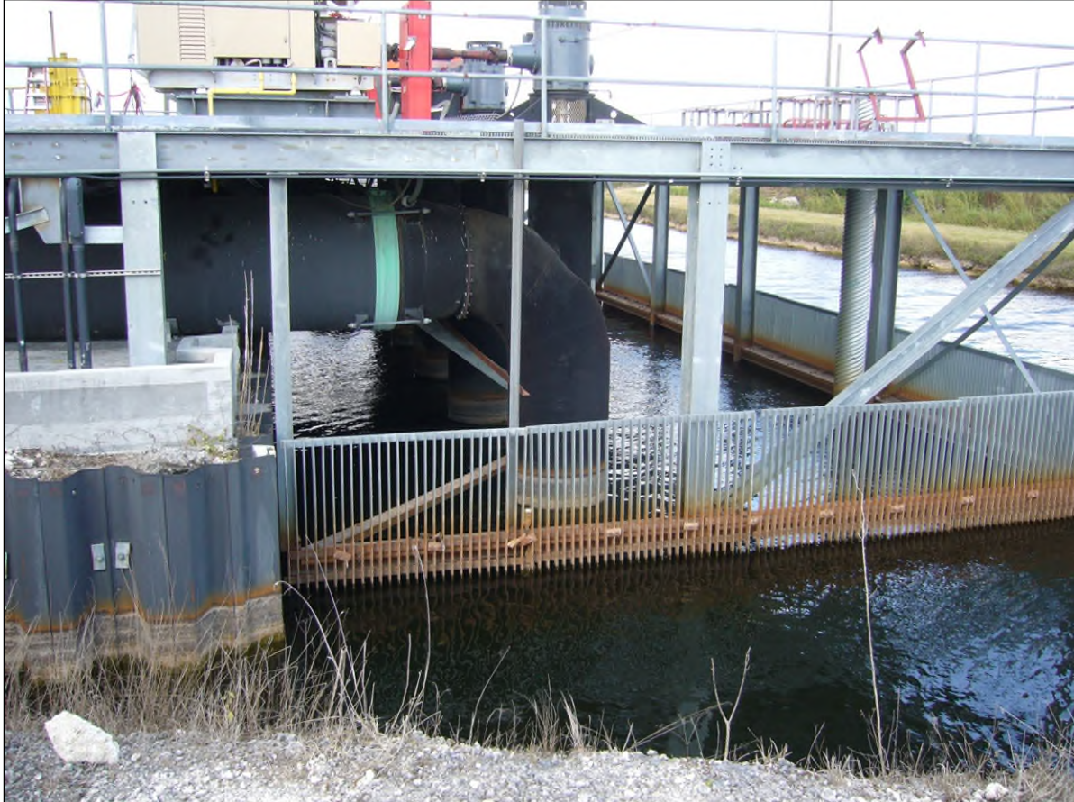
Figure G4. Inlet structure for pump station S332B
