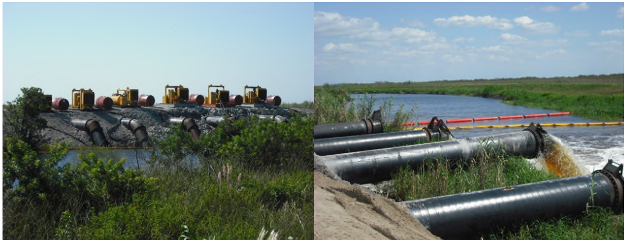
Figure G1. Temporary pump station at S-6 (head water at left, tail water at right)
