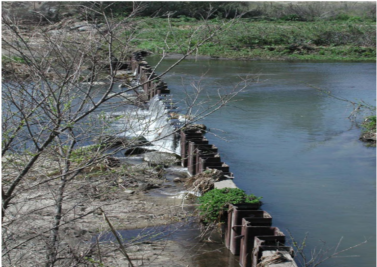
Figure E1. Sheet pile weir in the Santa Margarita River (from USBR, 2004)
