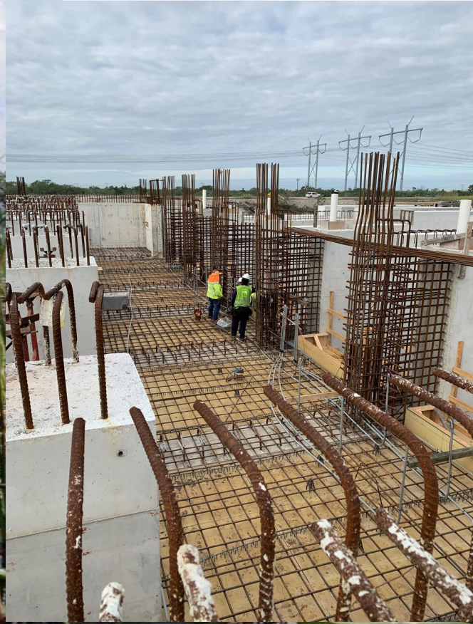
G-782 Pipe Gallery
