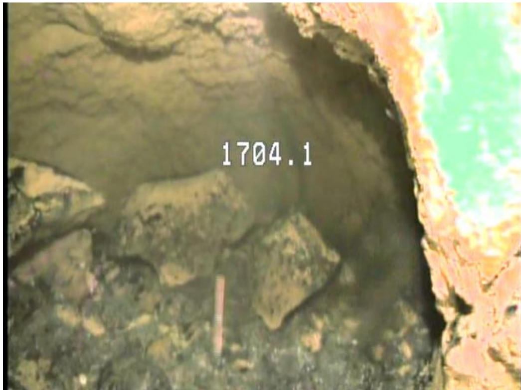
Figure 4-8. BHV view of cavity in OSF-109 with flow into borehole (cloudiness in center of photo)
