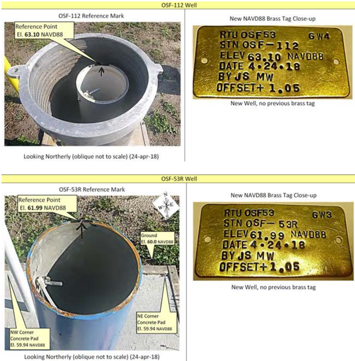
Figure 4. Completed wellheads showing measuring point elevations and their reference locations for depth-to-water measurements for wells OSF-112 and OSF-53R.
