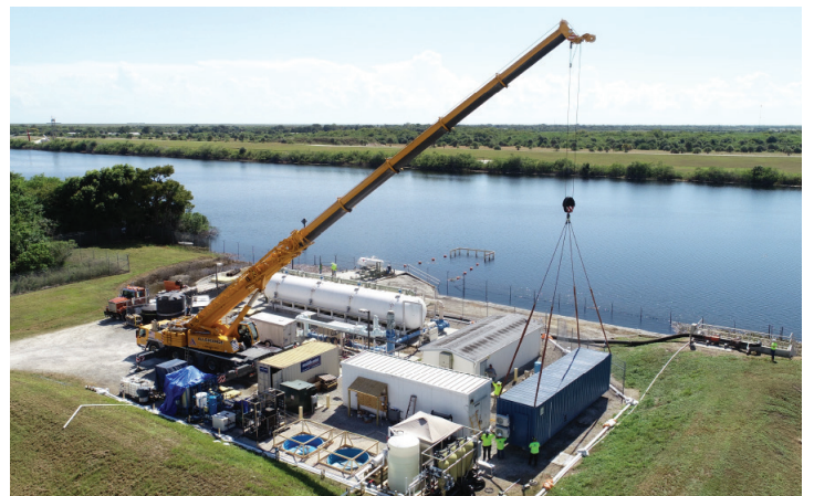
Existing Kissimmee River ASR well site (photo by SFWMD).
