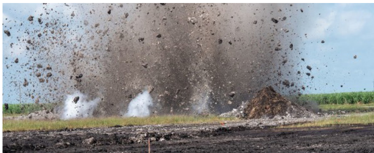
Figure 2. Blasting for a canal at the EAA Reservoir Project site on August 28, 2020. (Photo by SFWMD.)
