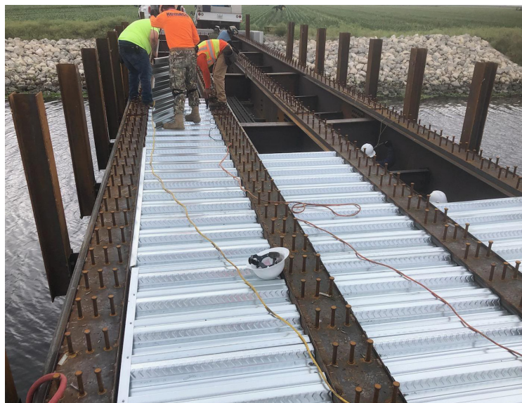
Figure 13. Installation of the Jet Farms Bridge, part of the Bolles East (L-16) Canal Conveyance Improvement. (Photo by SFWMD.)
