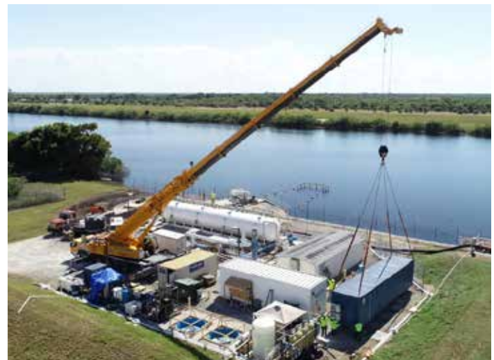
Existing Kissimmee River ASR well site (photo by SFWMD).
