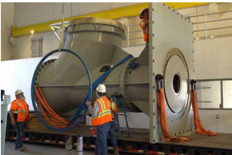
Installation of a New Pump at a Caloosahatchee (C-43) Reservoir Pump Station (photo by SFWMD).
