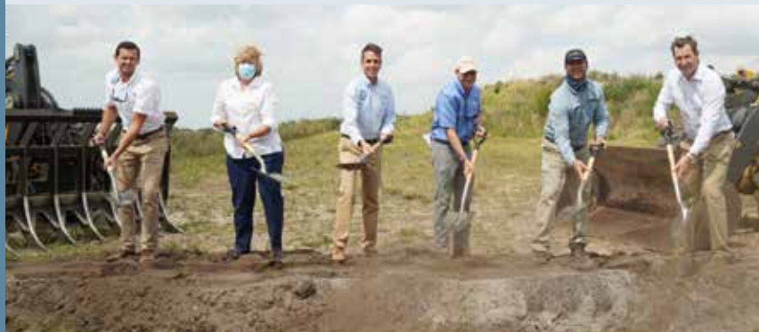
Groundbreaking of the C-139 FEB (photo by SFWMD). L-R: FDEP Southeast District Director Jason Andreotta, Mayor of Clewiston Kristine Petersen, SFWMD Executive Director Drew Bartlett, SFWMD Governing Board Chairman Chauncey Goss, County Coalition Chairperson Karson Turner and Andres Mendoza, President of Condotte America.
