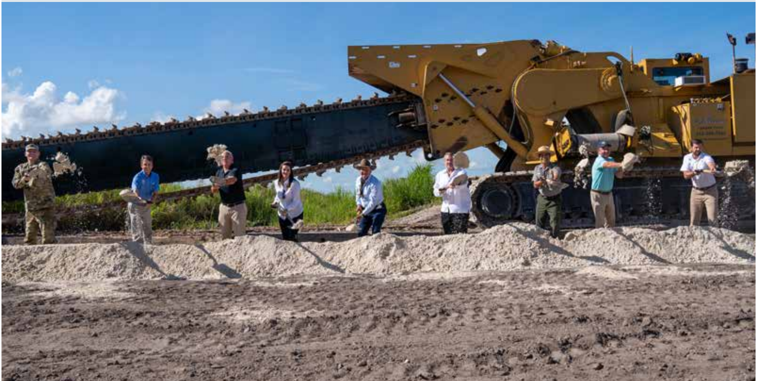
Breaking Ground on Underground Wall to Support Everglades Restoration (photo by SFWMD). L-R: USACE Jacksonville District Lt. Col. Todd Polk, SFWMD Executive Director Drew Bartlett, Congressman Carlos Gimenez, Lt. Gov. Jeanette Nuñez, SFWMD Governing Board Member Ron Bergeron Sr., Miami-Dade County Board of County Commissioners Chairman Jose "Pepe" Diaz, Superintendent of Everglades and Dry Tortugas National Parks Pedro Ramos, CEO of the Everglades Foundation Eric Eikenberg, and FDEP Southeast District Director Jason Andreotta.
