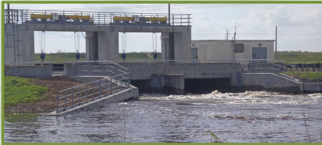
STA-1W G-303 gated structure
