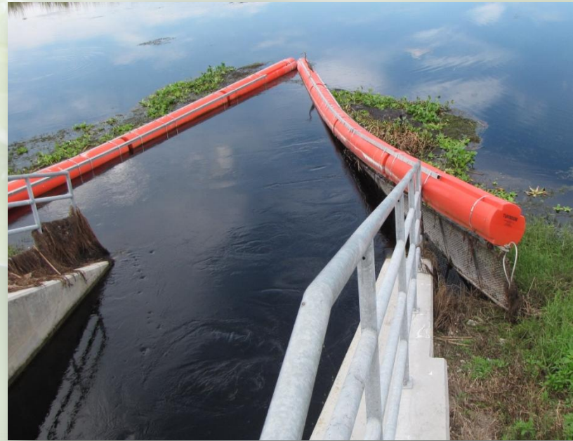
STA-1E Cell 3 outflow structure S-367A vegetation TuffBoom® buckled due to high flows. Vegetation remaining on the railing on left indicates elevated water levels.
