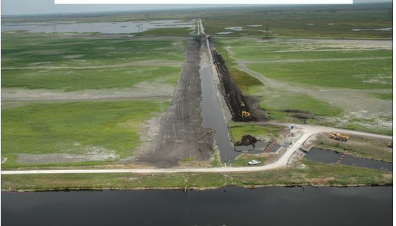
STA-1W Cell 4 removal of flow obstruction
