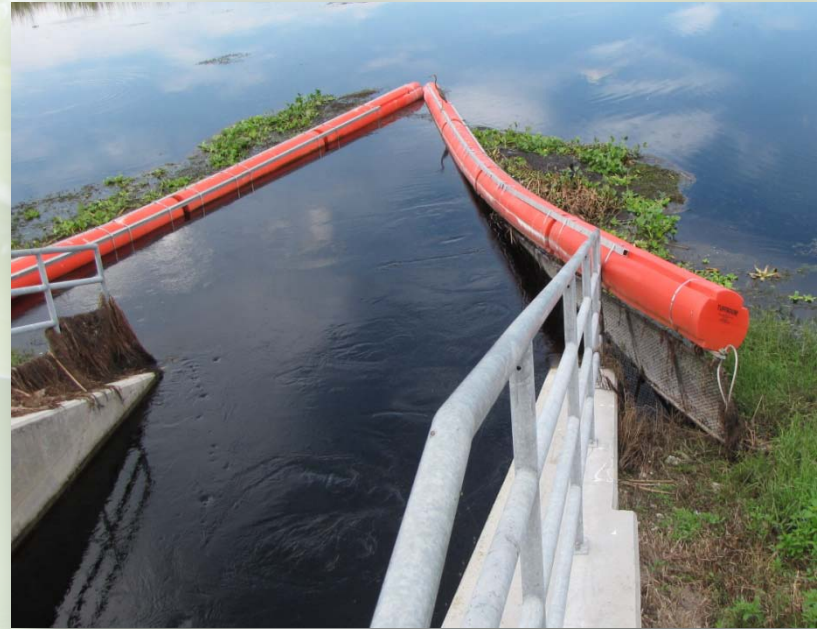
STA-1E Cell 3 outflow structure S-367A vegetation TuffBoom® buckled due to high flows. Vegetation remaining on the railing on left indicates elevated water levels.
