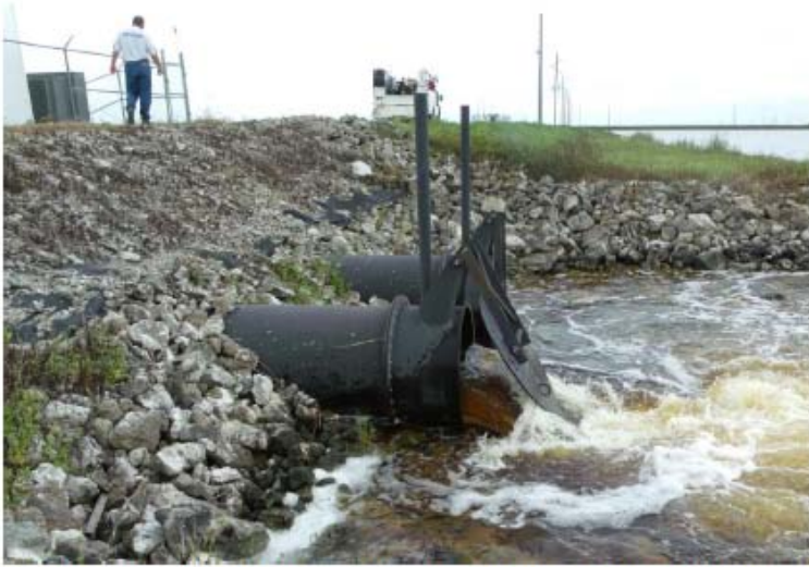
Figure 2. Discharge pipes shown with Pump #2 operating under 222 RPMs.
