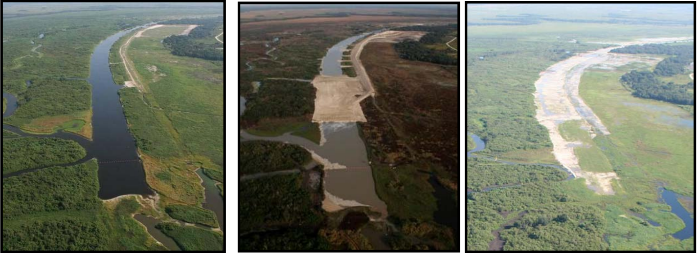
The major construction work for the restoration is being completed by contractors for the U.S. Army corps of engineers, it involves re-establishing the historic river channels, removing water control structures, and backfilling the C-38 canal that has diverted the waters of the floodplain since the 1960s.
