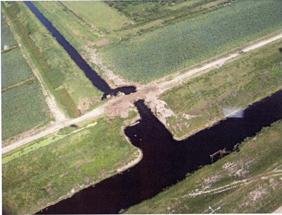
Breach at intersection of ALICO Canal and L-2 Canal – Looking northwest between Basin 26-323-05 (upper right) and Basin 26-310-03 (upper left) and Basin 26-310-01 (lower right)
