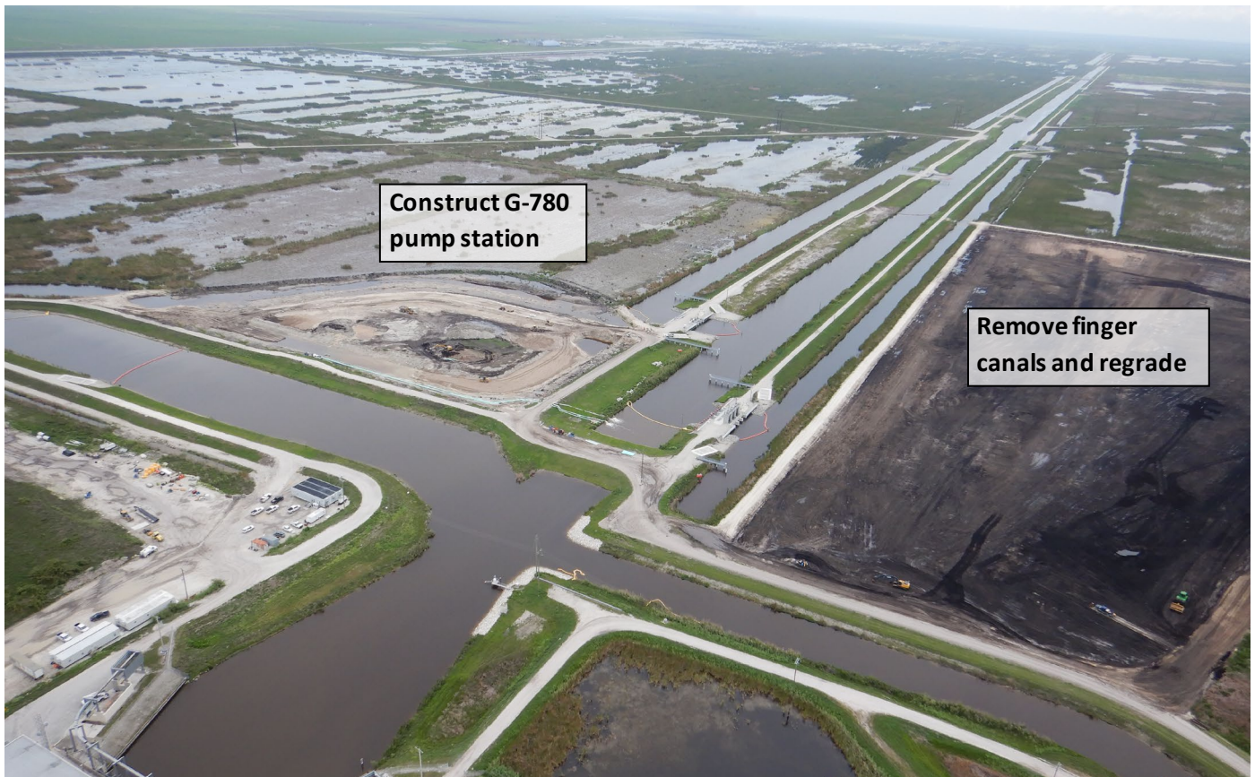
Aerial view of the south end of STA-1W, looking north. In the center right, the removal of finger canals and regrade of 50 acres in Cell 3. In the center left, the ongoing construction of G-780 pump station for Expansion No. 2.
