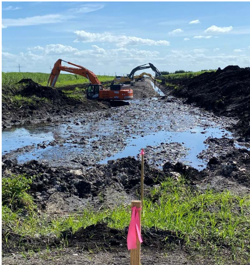
Eastern view of Segment 4 farm ditches and farm road replacement (G-341 Related Conveyance Improvements). Image depicts muck removal down to rock layer prior to placement of farm road and canal levee.
