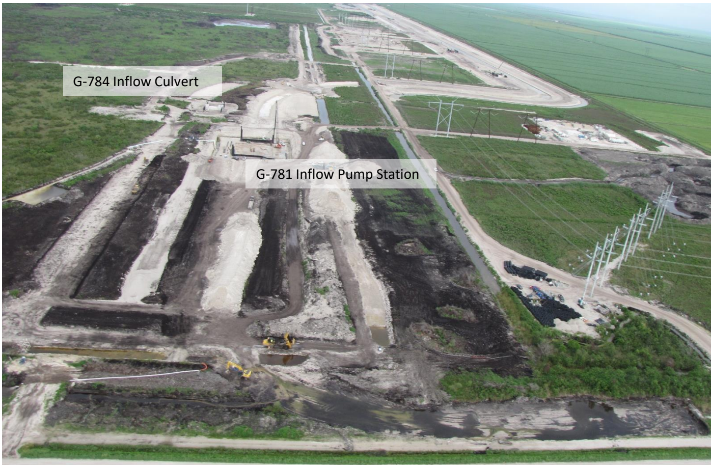
Westward aerial view of the STA-1W Expansion #2 Project. Image shows construction of G-781 Inflow Pump Station and G-784 Inflow Culvert in Cell 9.
